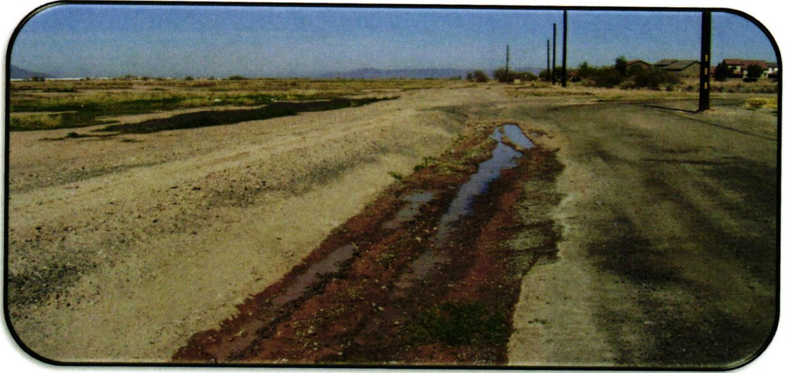
Figure 5: Water Retention in Street in Area Scheduled for Retention Basin
